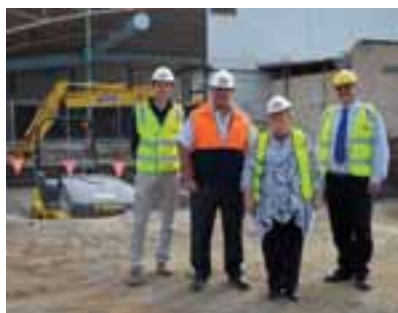
Excavation for the new warm water program pool. Left to right: Russell Whiteford, Bluewater Fitness Centre Manager, Henry Bongers, BDH Constructions, Cr Lyn Russell, Mayor and Cr Brian Crook.
