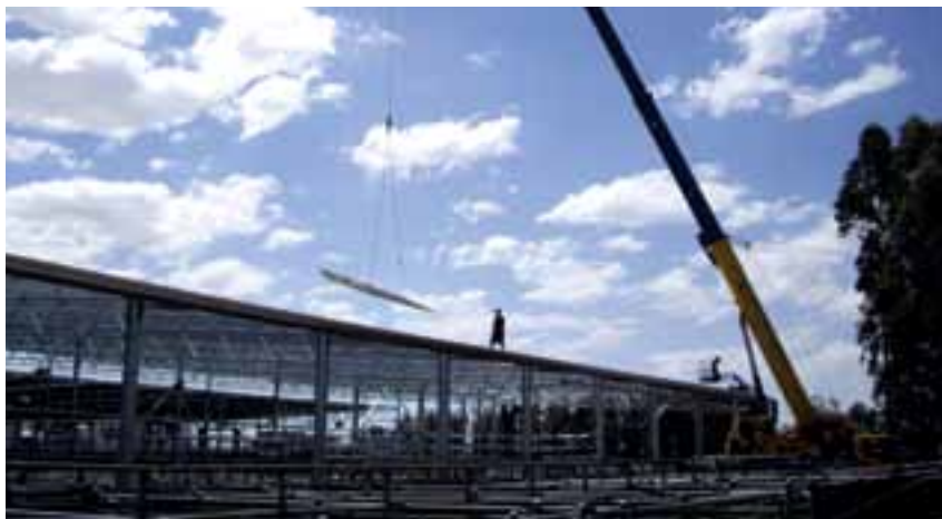
Occupational Health and Safety was carefully managed during construction of the roof over the Colac Regional Saleyards.
