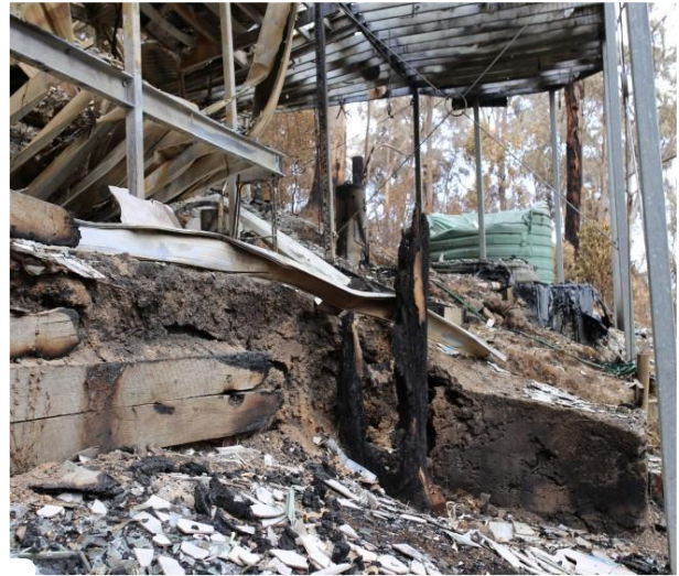
Figure 22: Remains of a retaining wall near a house
