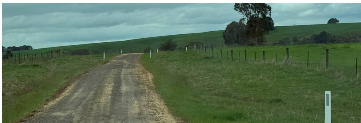
Figure 81 - Existing condition of Middle Murroon Road
