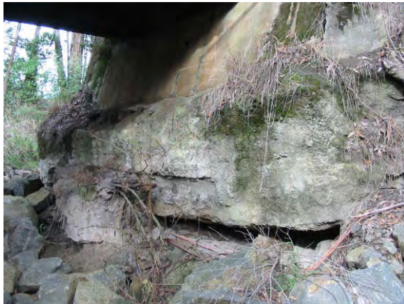
Undermining of Concrete Abutment
