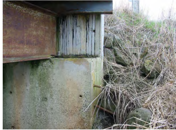
Missing Concrete Wingwall
